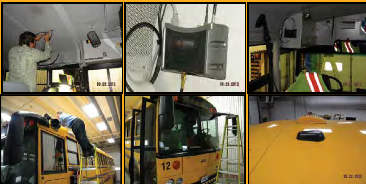
Wi-Fi and GPS tracking solutions being installed on local school buses by Palmer Wireless in October, 2012
